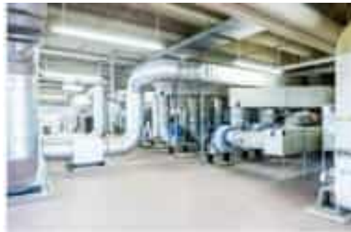
Figure 190 : Exemple des dispositifs techniques Source: https://fr.depositphotos.com/126164190/stock-photo technical-room-with-exhaust.html
