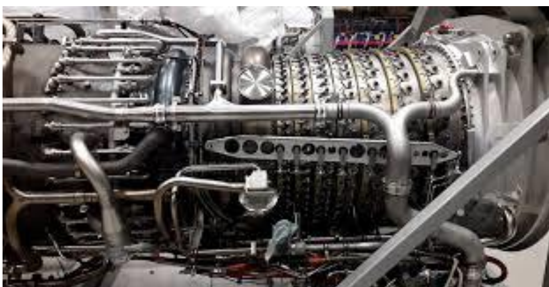
Figure II.19 PGT25 Gas Turbine Air Compressor (Company, 2025)
