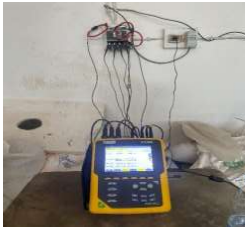
Figure III-8 Measuring instrument Electrical network analyzer QUALISTAR
