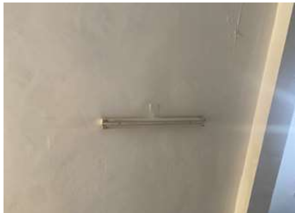
Figure III-17 Malfunctioning Lamps on Lighting Conditions
