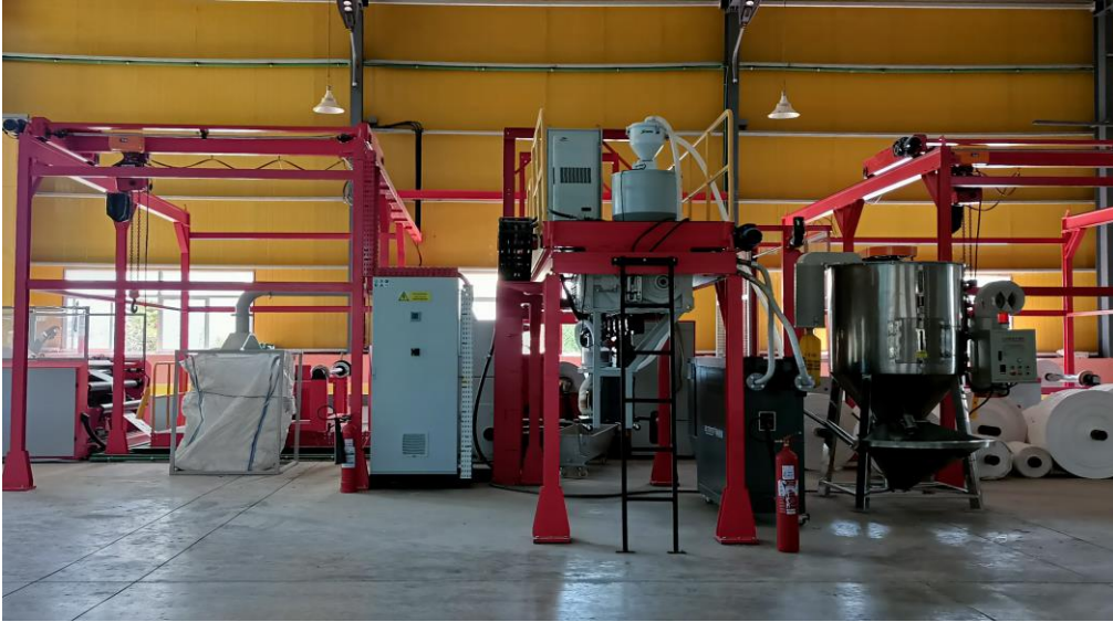
Figure II. 13 : Machine de lamination
