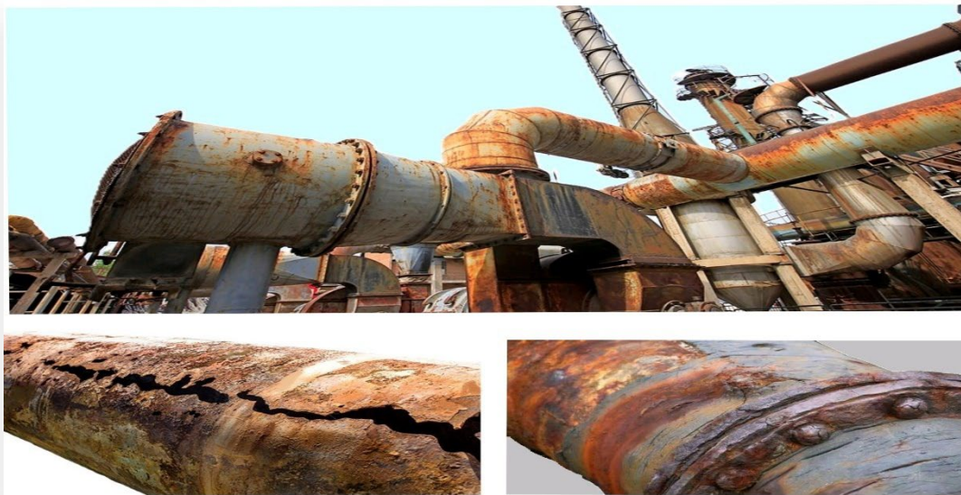
Figure 12: Corrosion on pipelines.
