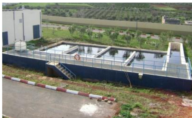
Figure III.8 : bassin de chloration.
