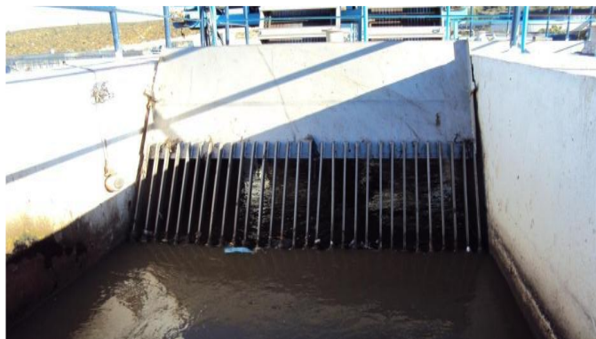
Figure III.3: Grille grossière manuelle (1unité).
