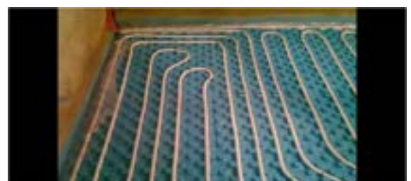
Figure 83: chauffage de hammam
