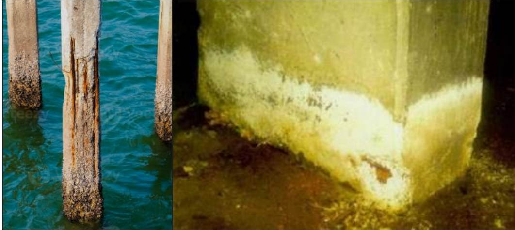
Figure 1. 22: pathologies due to sulfate attack [32]
