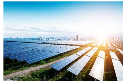
Figure 23: des panneaux photovoltaïques.
