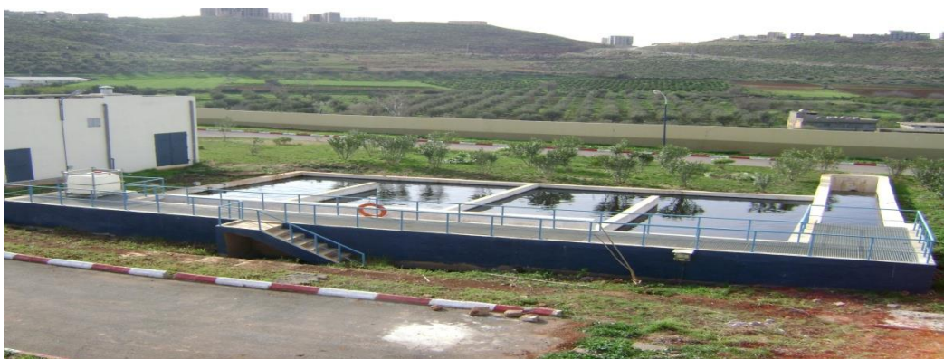
Figure 30: Bassins de chloration
