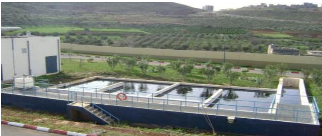
Figure IV. 12: Bassin de chloration [53].
