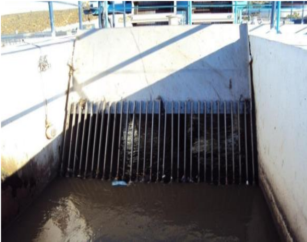
Figure IV. 3: Grille grossière manuelle [53].
