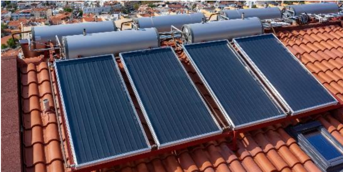
Figure I.8: Thermal solar energy [14]
