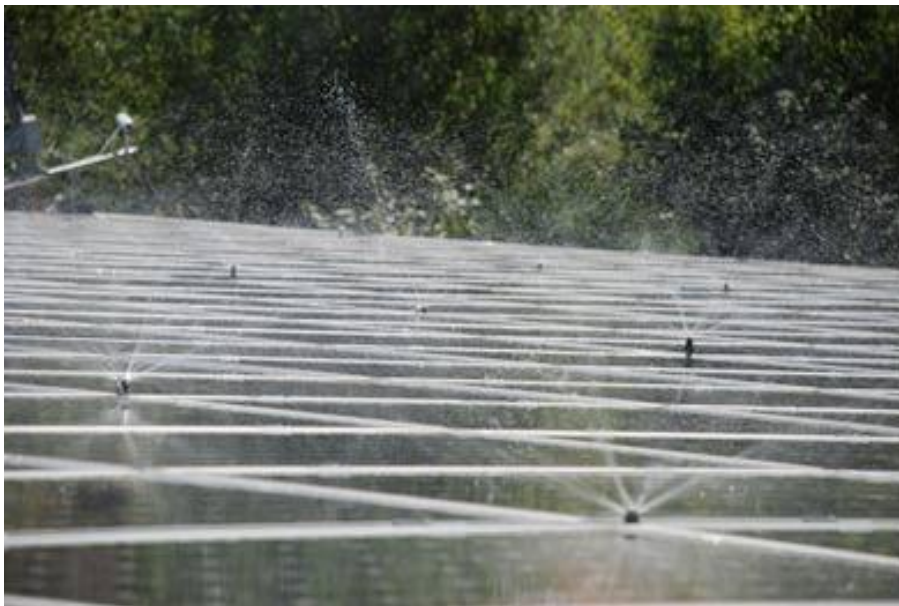
Figure III. 13: SUNI Brain sprinkler cooling system [42]
