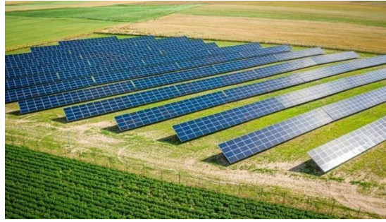
Figure 68 Peneaux photovoltaïques – source google photo -
