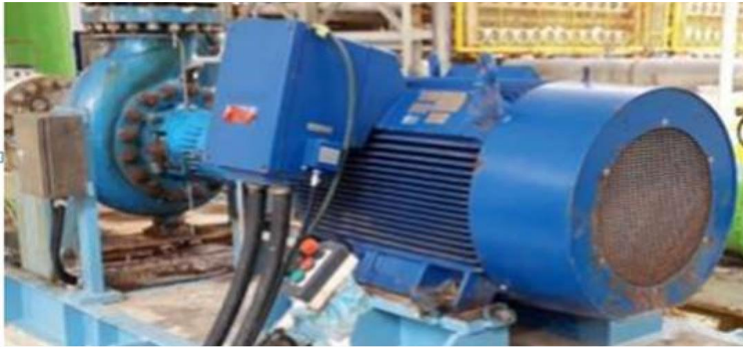
Figure 35 : Pompe Booster (origine ;2025)
