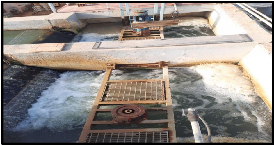
Figure.13: les bassins de Coagulation – Flocculation.
