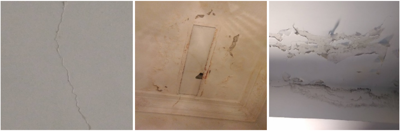
Figure I.3 : Examples of problems caused by moisture.
