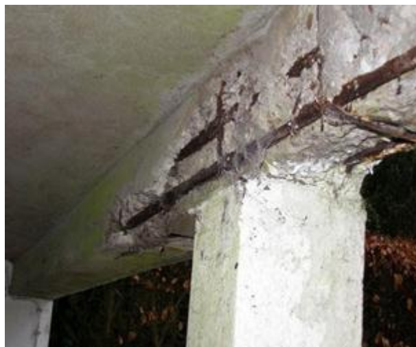
Figure 3.3. Corrosion des armatures [45]
