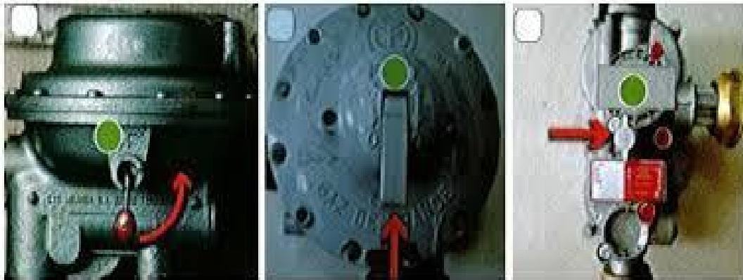
Figure I.12: Vanne de coupure gaz
