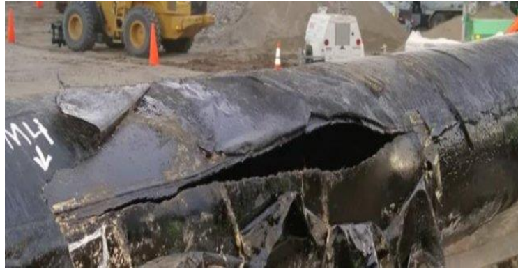
Figure I.2 : Fissuration du pipeline [2]
