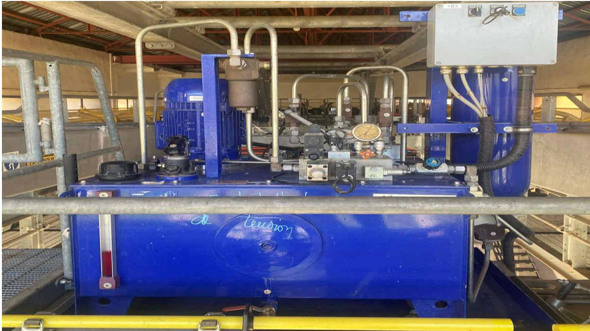
Figure 38 Centrale hydraulique [Photo personnelle]
