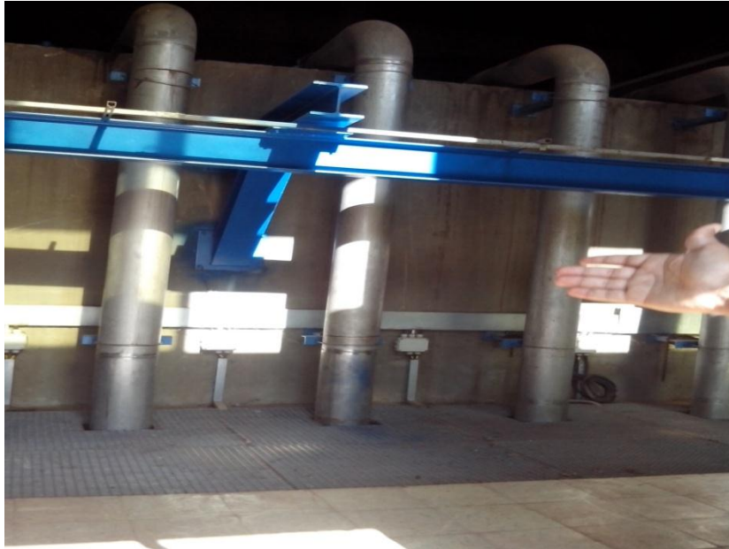
Figure III.8: Poste de relevage
