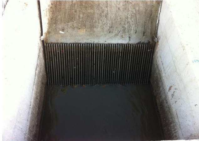
Figure III.5: Photo de la grille manuelle de by-pass
