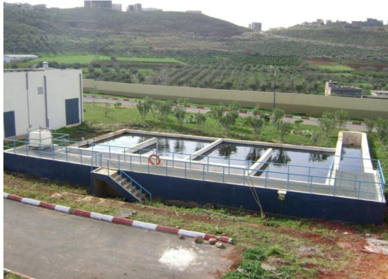
Figure III.11: Photo du bassin de chloration
