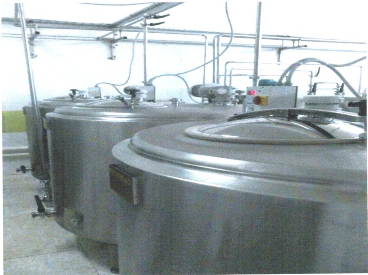
Figure 27 : cuves de maturation
