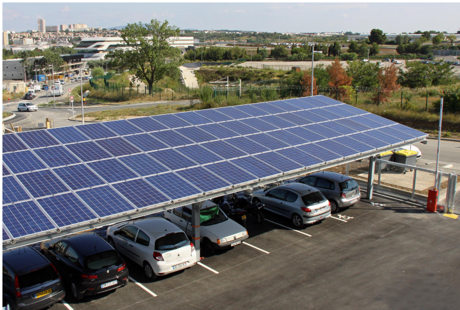
FIGURE 1.23: Ombrière photovoltaïque de parking.
