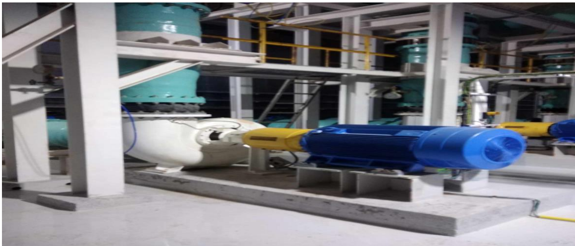
Figure 16 : Pompe aspirante (origine 2024).
