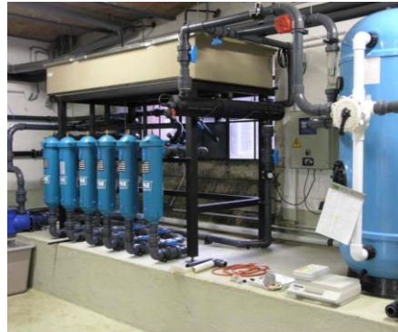
Figure 120: station de filtration Source: google images
