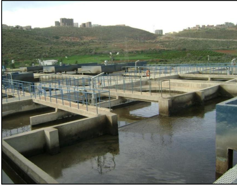
Figure 11 le bassin de la nitrification/dénitrification.
