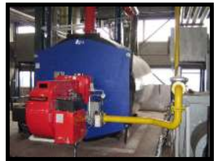
Figure 365 Chaufferie Eau Chaude
