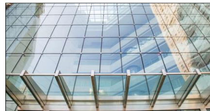
Figure 131 : vitrage photovoltaïque Source Google photo
