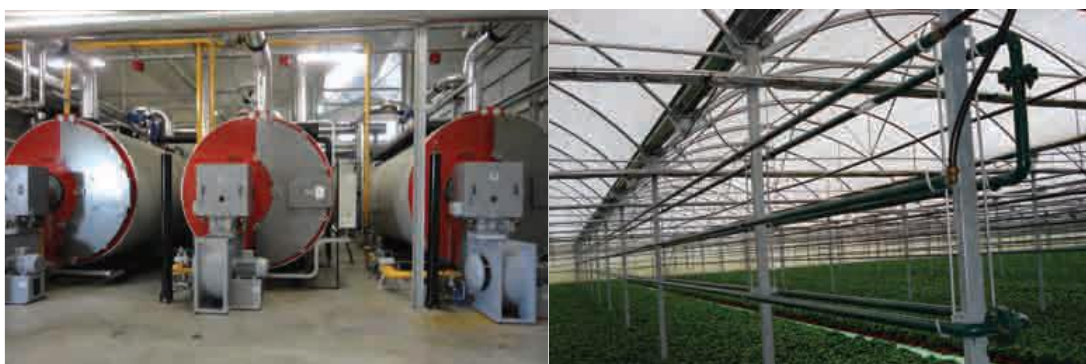
Figure 1.13 Central boiler (left) and heating pipes for dissipating the produced heat (right)
