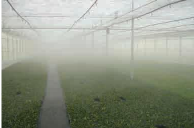
Figure 1.11 Fog system used for greenhouse cooling
