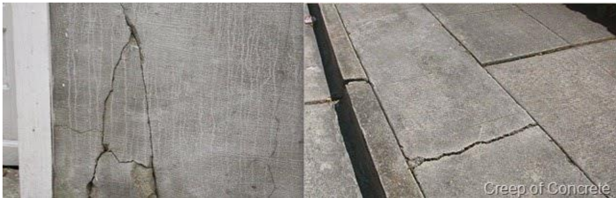
Figure 1-11 Cracked concrete structure due to creep. (Online Civil Engineering, n.d.)
