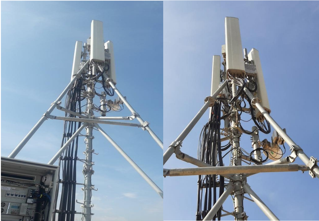
Figure 4.4 : Antenne Node B
