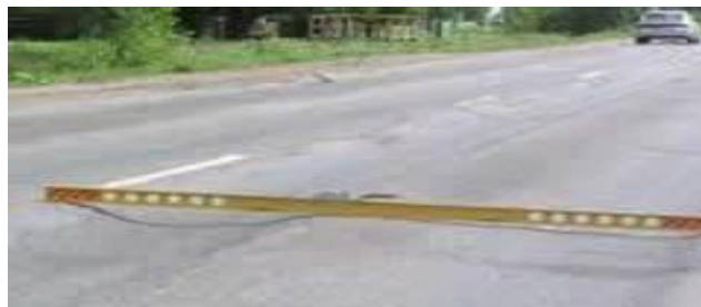
Figure II.1 - Ornières (Déformations)- depositphotos.com-
