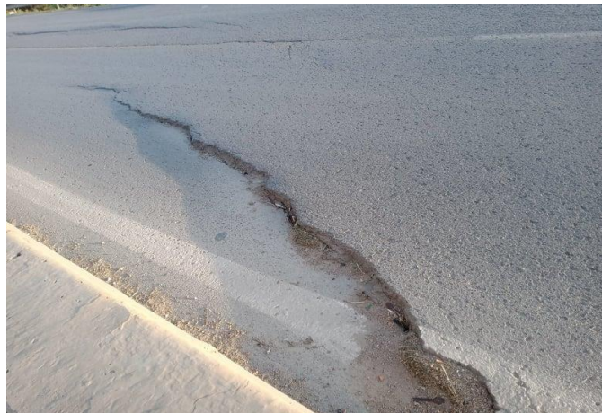
Figure II.13 fissure longitudinale (photo de notre expertise le 05/04/21)
