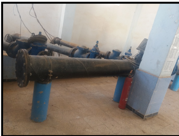
Figure IV.16: Les pompes de la station de relevage.
