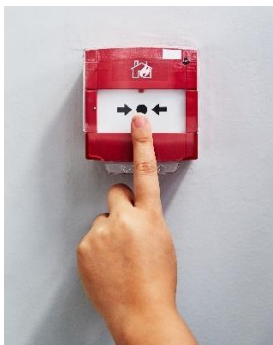
Figure : Alarme incendie
