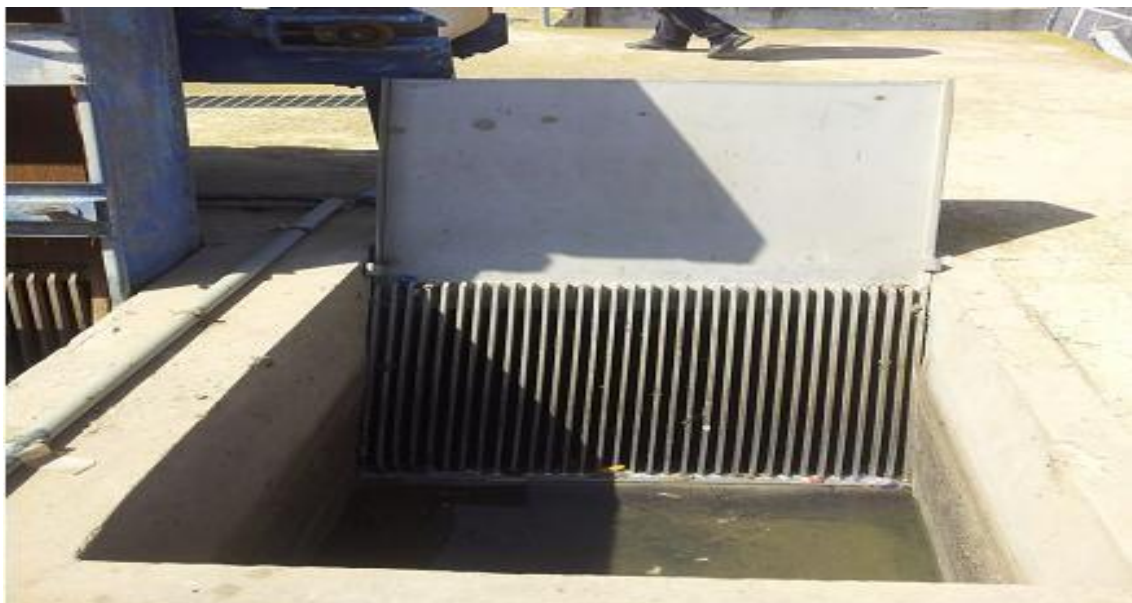
Figure II.34. Grille manuelle (Ain Bouchakif)
