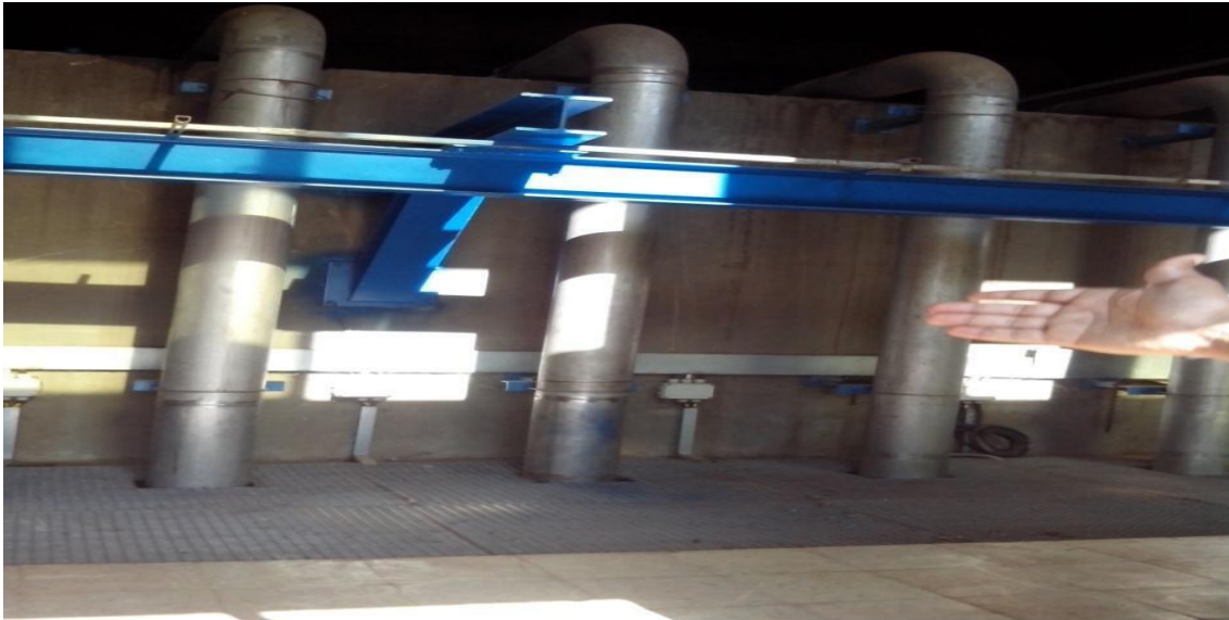
Figure II.11 Poste de relevage (Terga)
