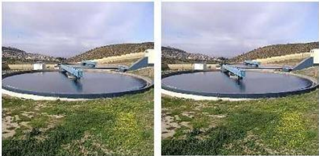
Figure II.25. Clarificateurs (Ain El Houtz)
