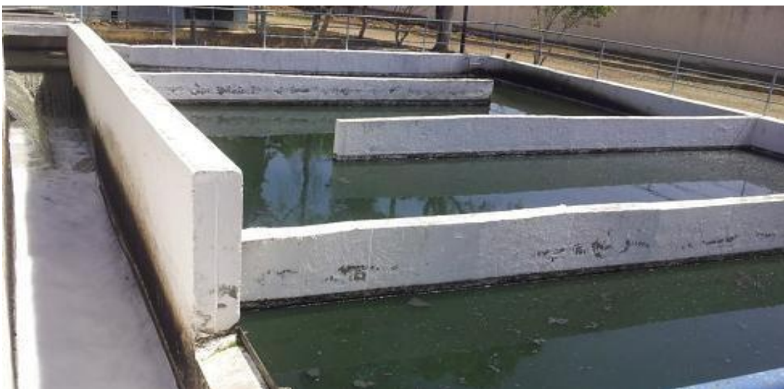
Figure II.38. Bassins de chloration (Ain Bouchakif)
