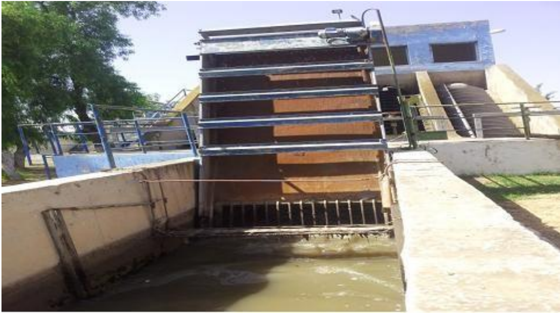
Figure II.31. Grille grossière manuelle (Ain Bouchakif)
