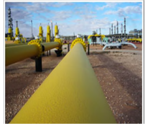
Figure 1 station de canalisation [3]
