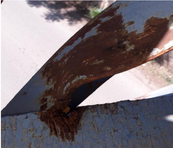
Photo.3.16 Propagation de la corrosion.
