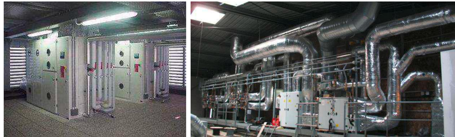
Figure 115 : Installation de ventilation
