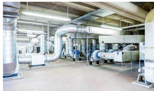
Figure 126. Exemple des dispositifs techniques (source : https://fr.depositphotos.com/126164190/stock-photo-technical-room-with-exhaust.html )
