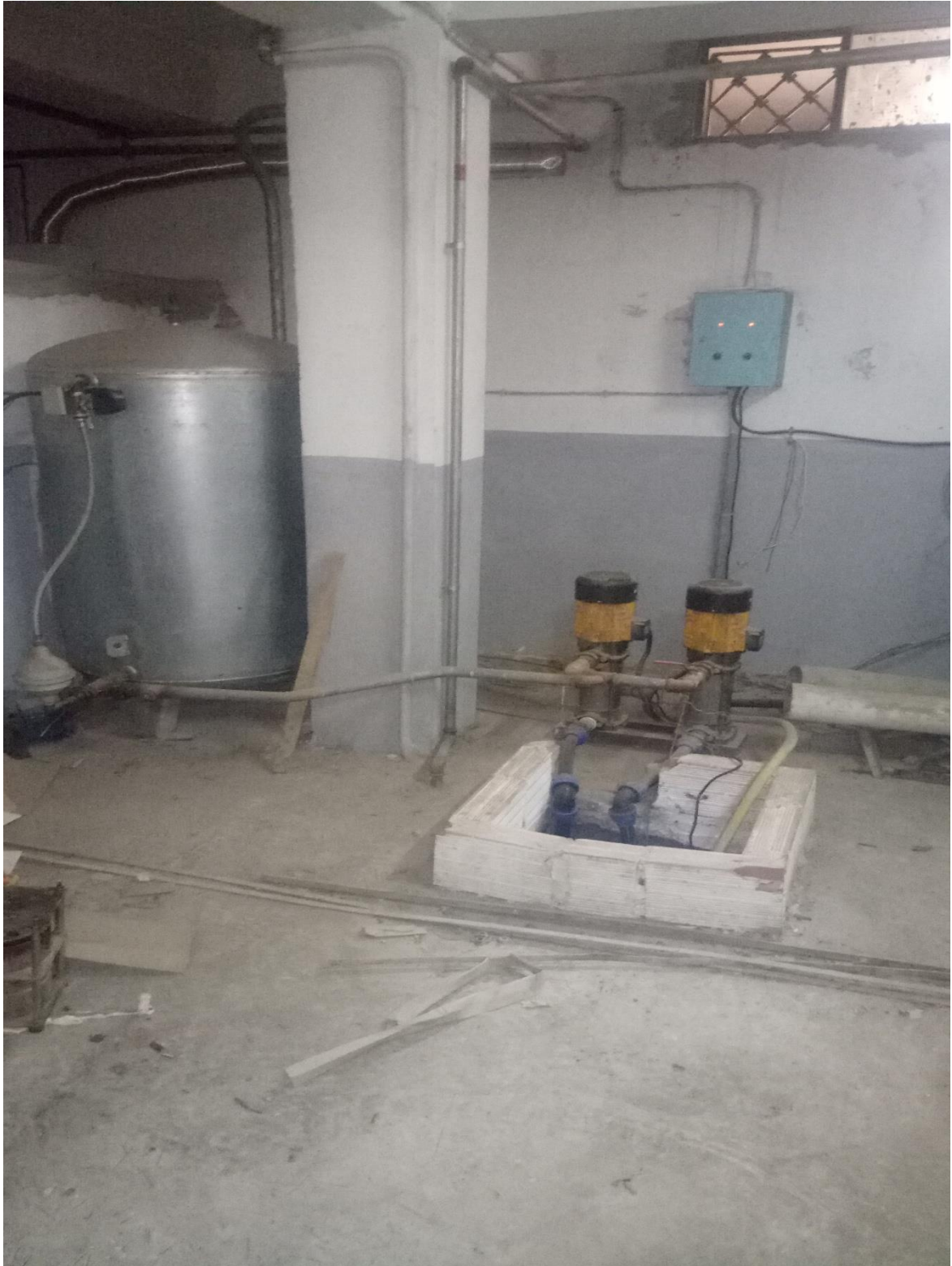
Figure 2-2 : Station de pompage
