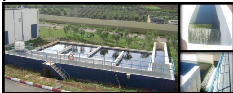
Figure 20: Bassin de chloration
