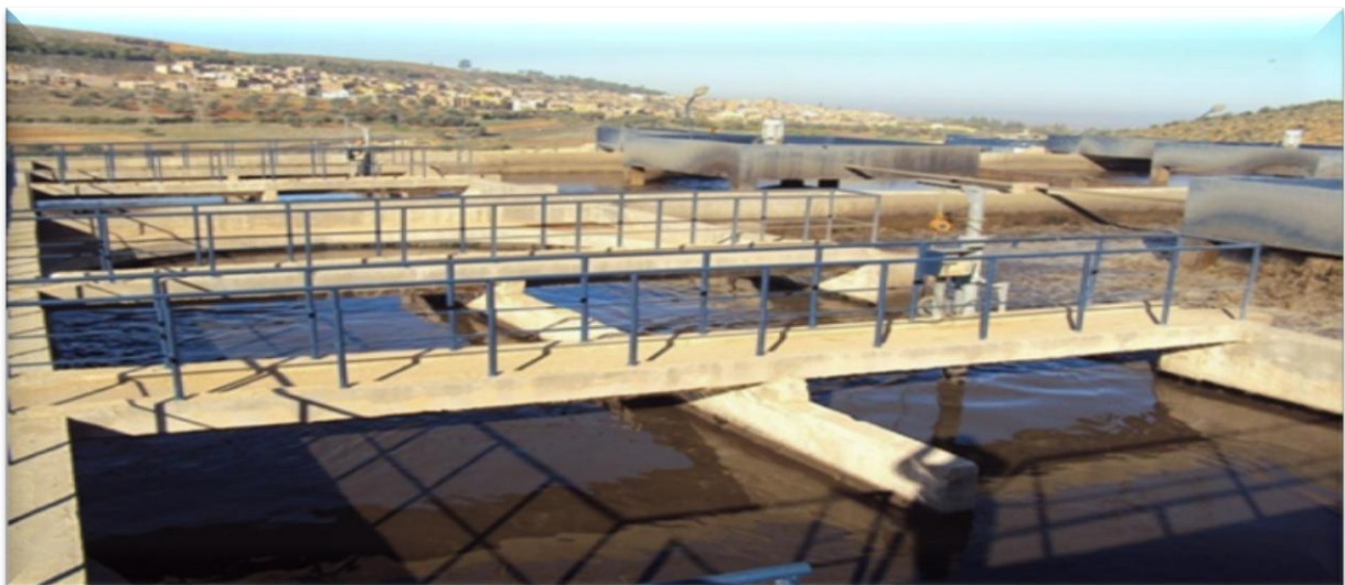
Figure II.13 : Bassin de nitrification dénitrification [30]
