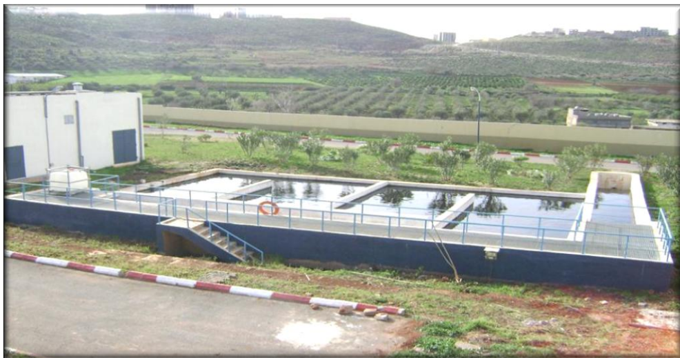
Figure II.16 : Bassin de chloration [28]
