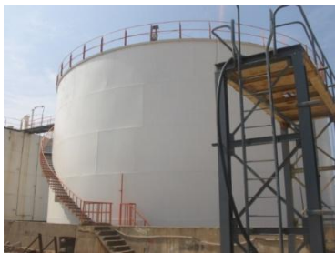
Figure07: Tank de stockage de H2SO4
