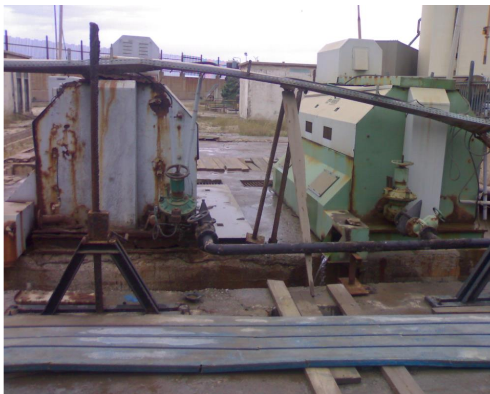
Figure III.11 : Filtres de la station
