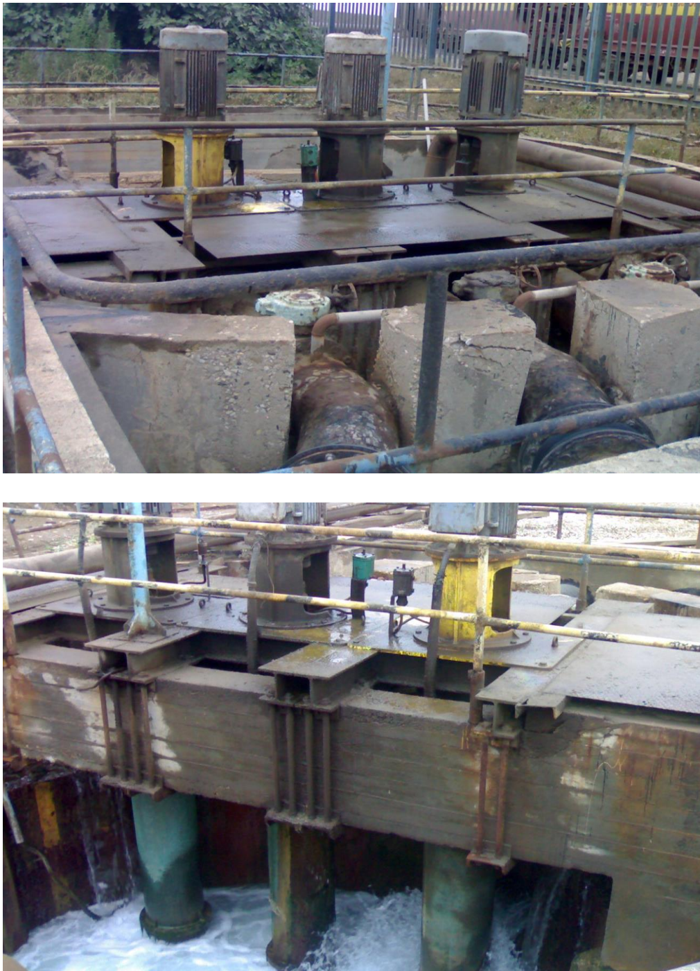
Figure III.12 : Pompes centrifuges de reprises
