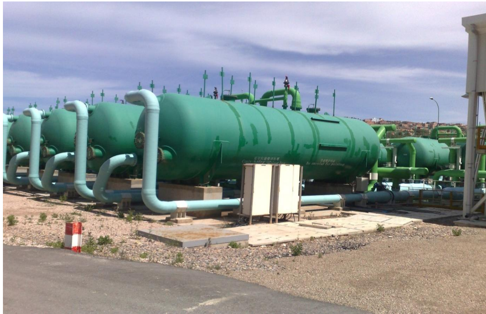
Figure III.9: photo des filtres multicouches
