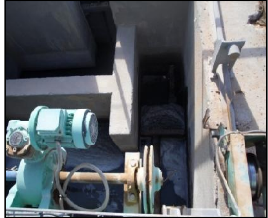
Figure III.13: Pont racleur de surface (27/05/2012)
