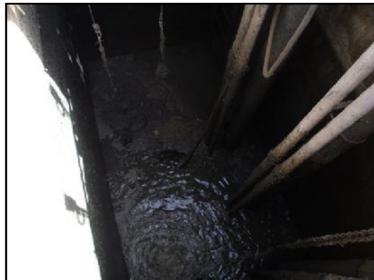
Figure III.7: La station de relevage (22/05/2012)
