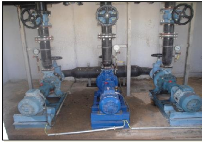
Figure III.11: Le Poste de Recirculation (14/05/2012)
