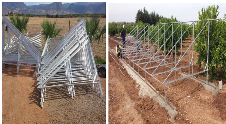
FIGURE III.2 – Supports des panneaux solaire
